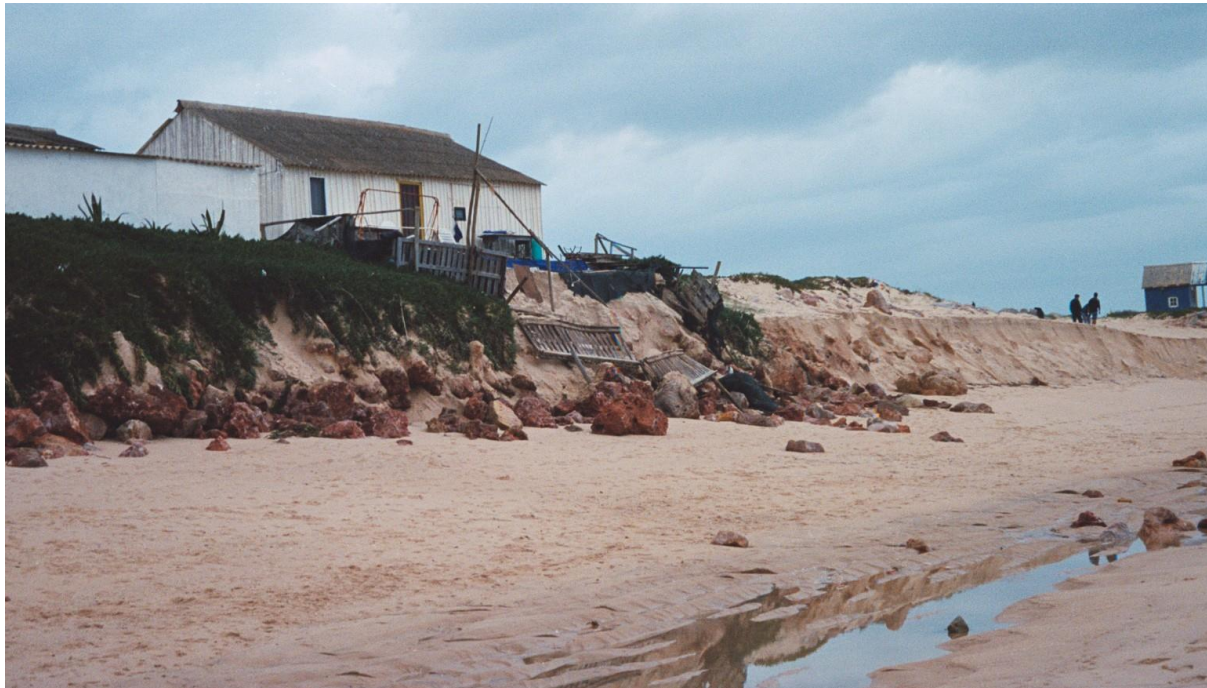
Figure 2.2 – House threatened by storm-induced erosion at Faro Beach in the winter 2003 (the house seen in the photo is the same as in Figure 2.1). Source: author’s photo.
