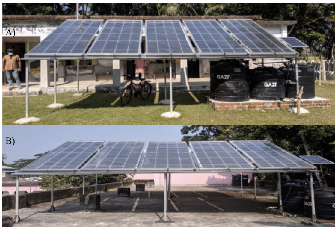
Figure 2.8 F CUBED panels with feed water, freshwater and brine tanks located in different places. A) Example of F CUBED panels installed on the ground. B) Example of F CUBED panels installed on a rooftop, example that Culatra will follow. (Source: Solar Water Purifier – Water purification systems, 2022).
