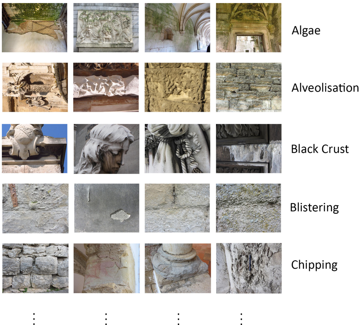
Fig. 2. Example of the deterioration patterns used for benchmarking.
