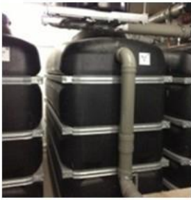
Rainwater harvesting system in Coventry (United Kingdom).
