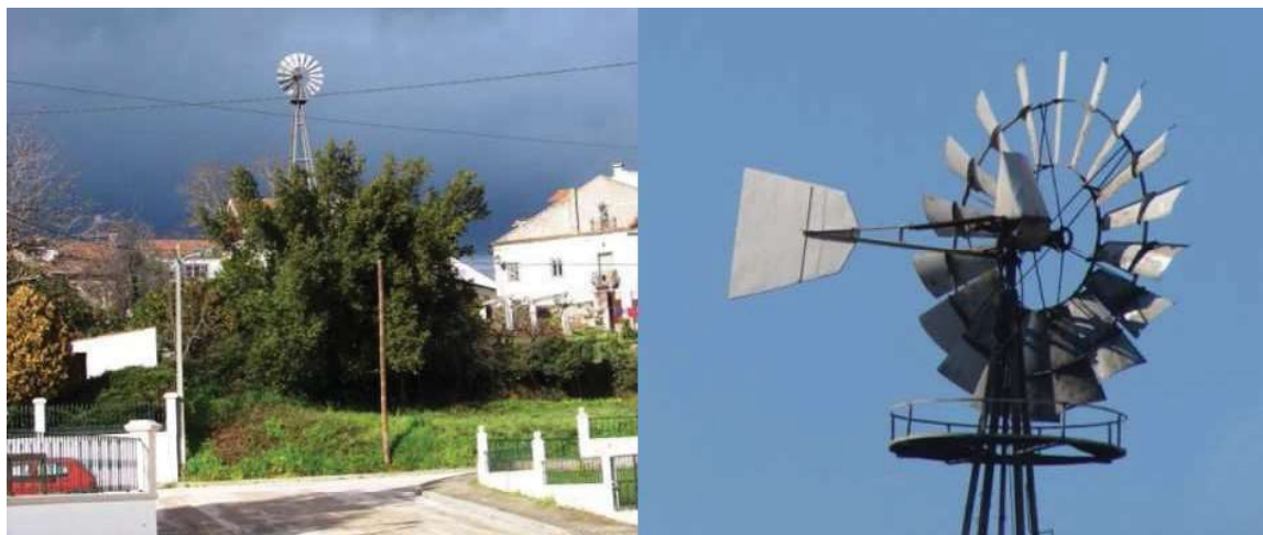
Figure 5. Wind powered water wells. Left: overview; right: detail (authors).
