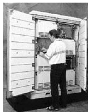
Foto 20 BSC – Base Station Controller
