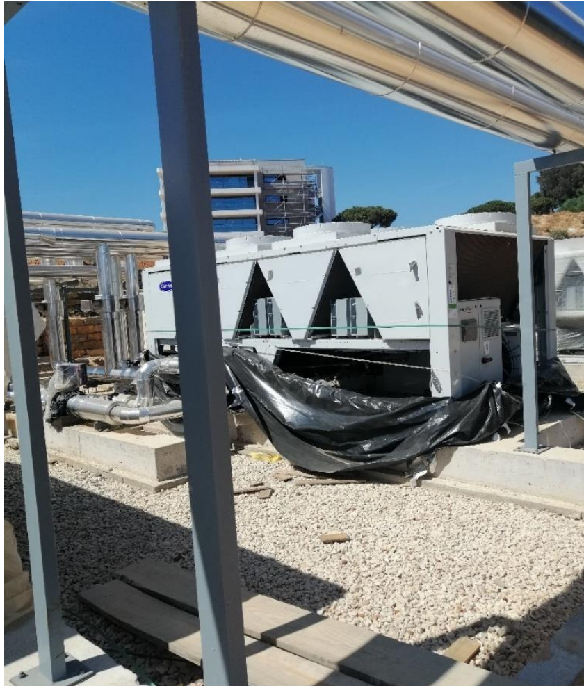
Figura 0.16 – Chiller – Central Exterior
