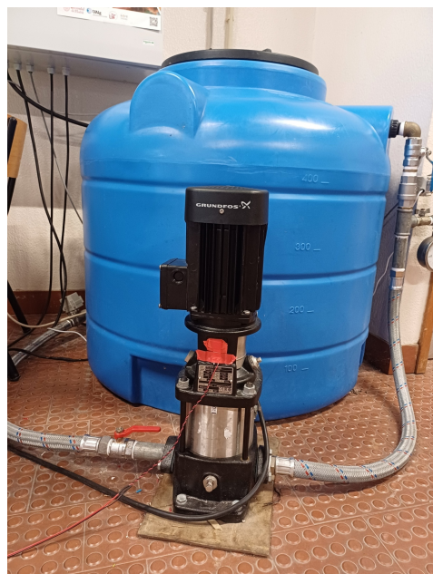
(a) Pump and reservoir
