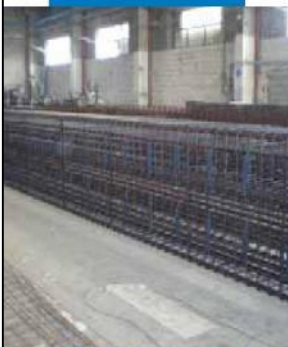
Mapeshield I welded to the reinforcement of a new beam in the construction of a dockyard quay
