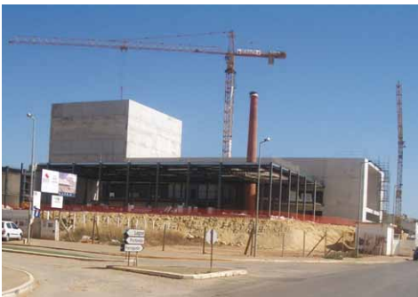
Figure 6. Pavilhão do Arade during construction - used by permission © Luís Loures, all rights reserved.
