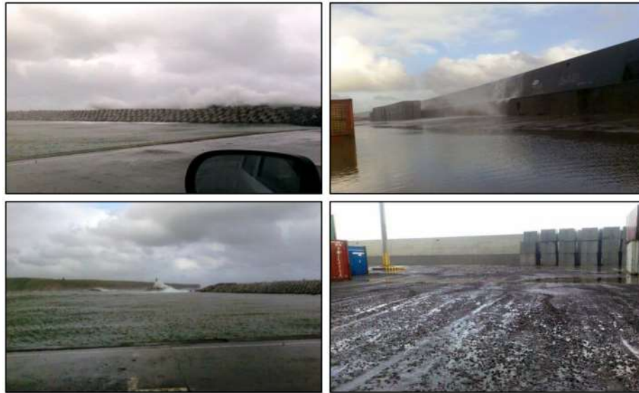
Figure 2.9-Damage and overtopping of the wave wall on the south breakwater protecting the container yard, leading to flooding of the yard during the storm event on January 24 th , 2007 (Source: Poseiro (2019)).
