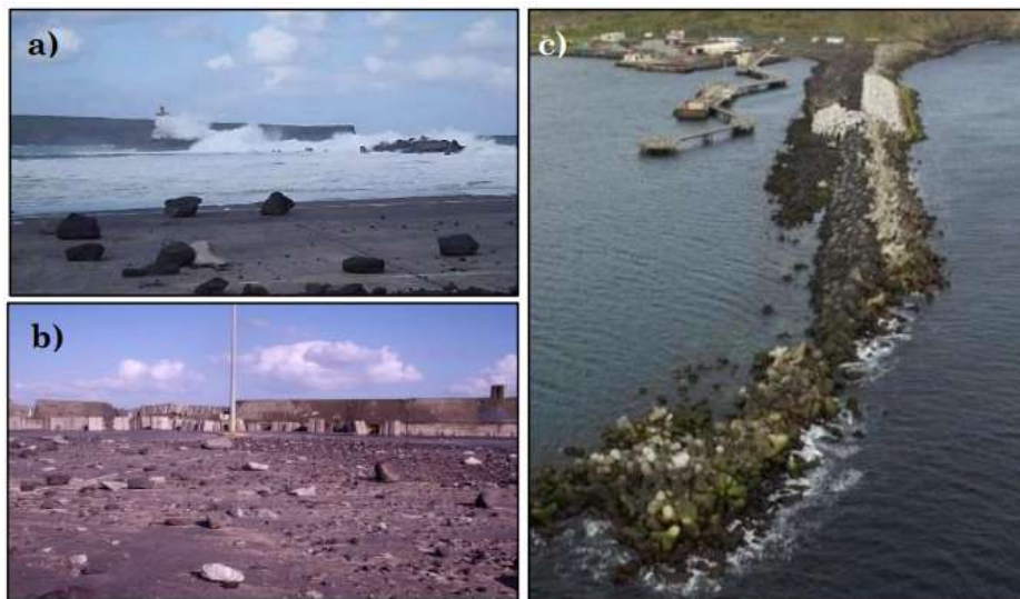
Figure 2.8- Damage to the south and north breakwaters, and the container yard in the storm on 26 th to 27 th February 2005 ( Source: Poseiro (2019) ).
