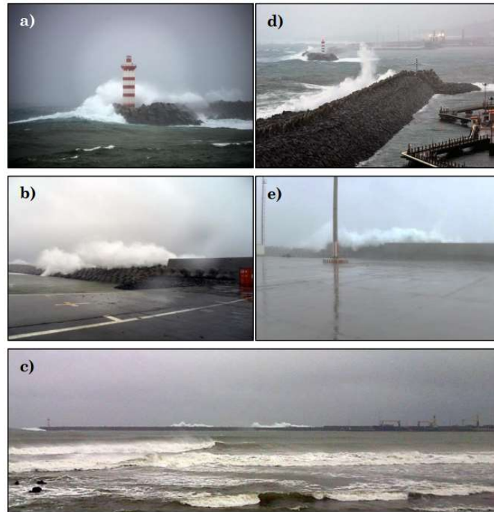
Figure 2.11- (e) Overtopping of south breakwater, flooding yard (a,b,c and e), and severe overtopping of the north breakwater (d)( Source: Poseiro (2019) ).
