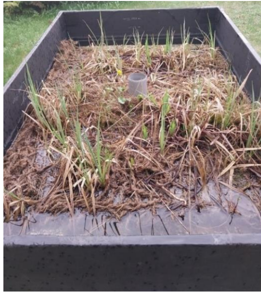
Figure 2.11. EPDM roof with standing water, Caxit and vegetation.
