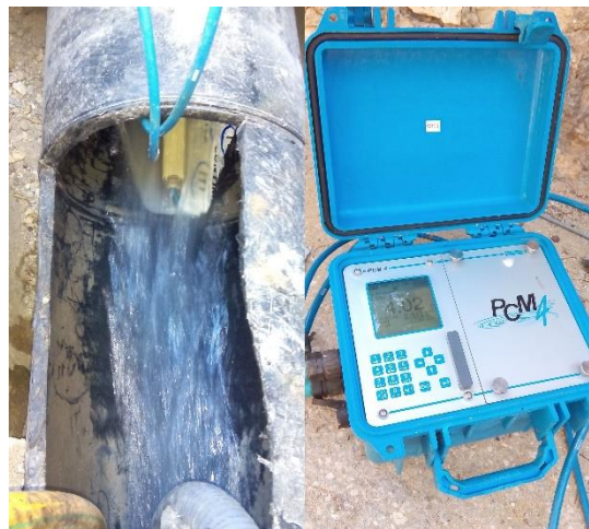
Figure 4.1. Equipment installed during the flow measurement campaign of Inatel outfall
