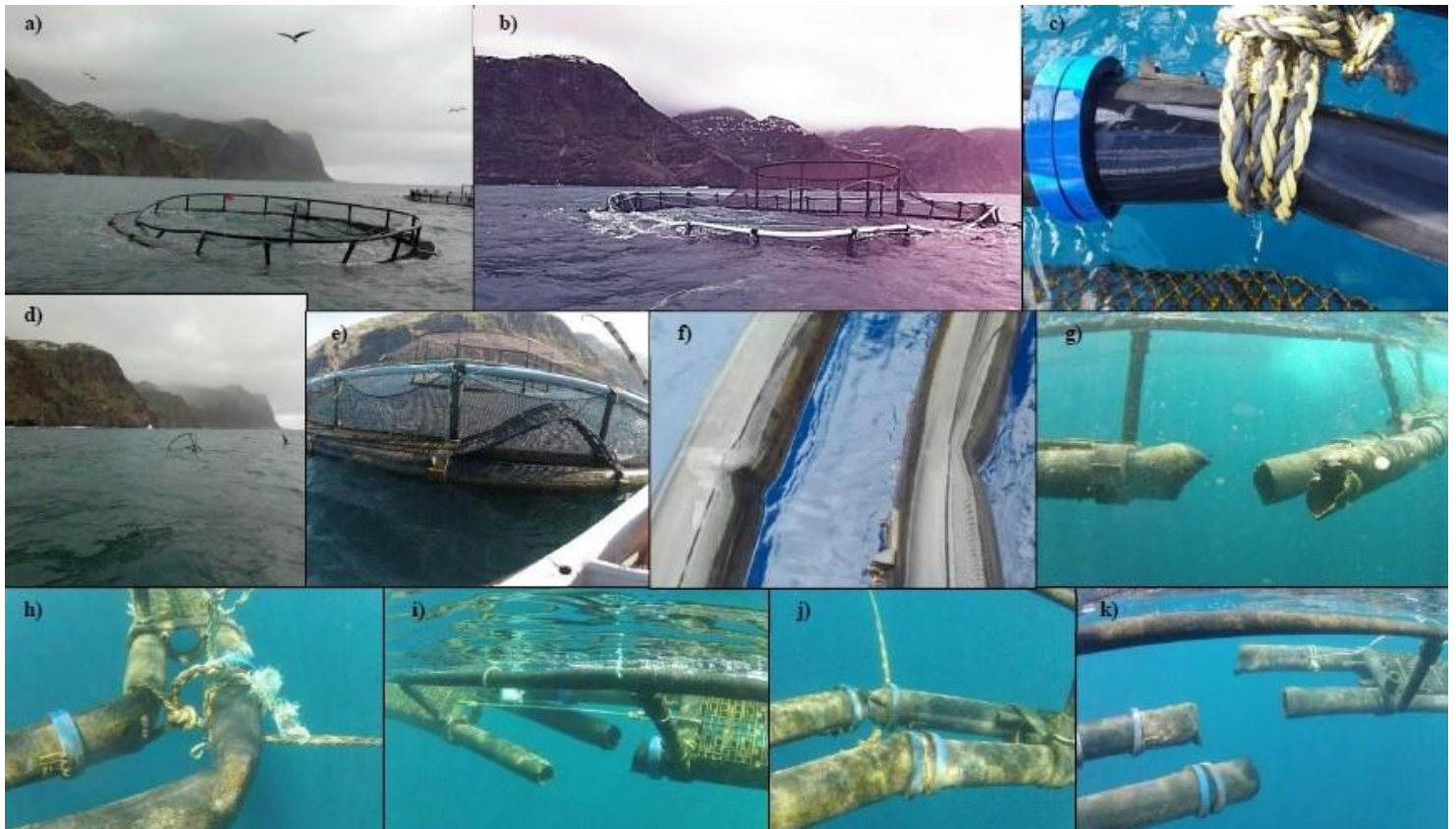
Figure 2.4 Damage at the fish farm in Ribeira Bava resulting from extreme weather conditions in February 2018: Deformation of the floating tubes (c, e, f, h), including strangulation and breakage of the floating tubes (g, I, j, k ), dislocation of the surrounding walkways (e), sinking of the net pen; with only the bird-protection net remaining at the surface, (d) and partial sinking of the net pen (a, b, e),© Aquabaia
