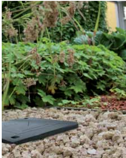
Up to about 40 l/m 2 of stormwater can be stored in the system build-up of an intensive green roof, .....
