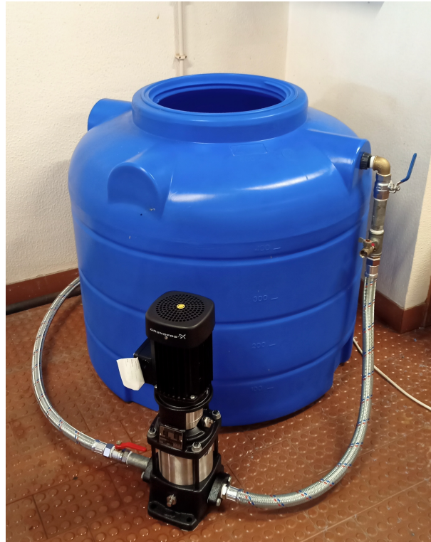
Figure 3.1: The hydraulic system, designed for the simplest possible real-world data acquisition.
