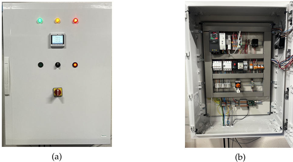
Figure 4.3: The new electric panel, closed (a) and open (b).
