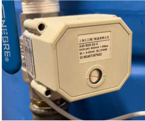
Figure 4.12: One of the 2 motorised valves, installed in the system.
