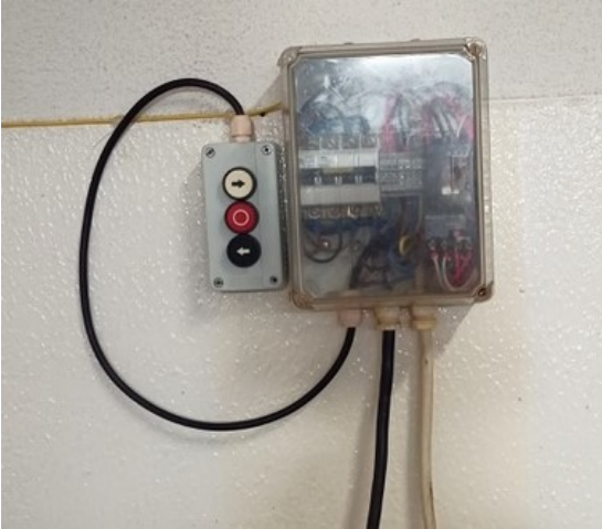
Figure 3.3: The first electric panel, designed for simple pump state commutation.
