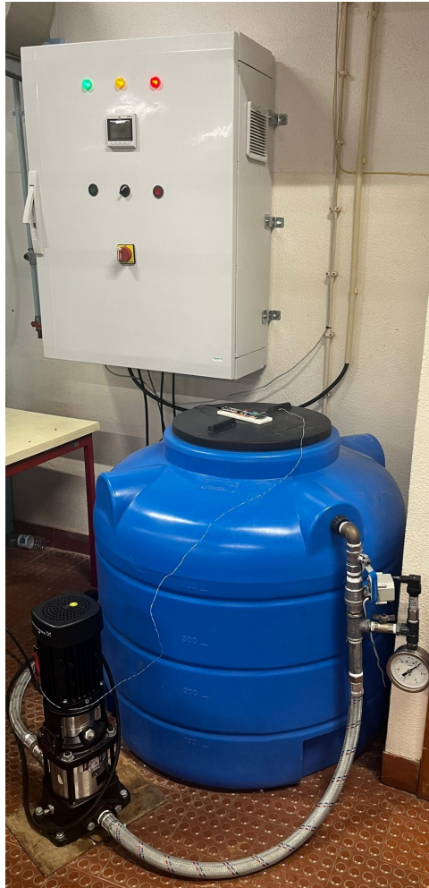
Figure 4.2: The automation system built in its entirety.
