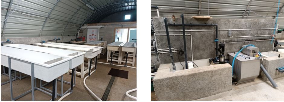
Figure 3.4: An assembled water circuit containing 7 troughs (200-300L) equipped with a reservoir, aquatic heaters, UV, particulate, & bio media filtration
