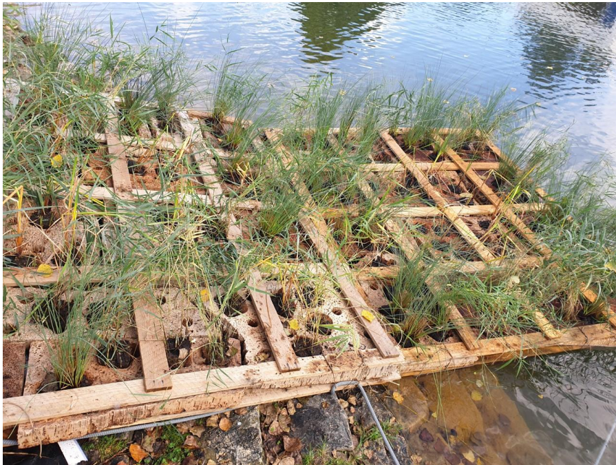
Figure 31. Island Design 3 being deployed in "the traditional way" due to crane defect (picture taken by author on 25.10.2022)
