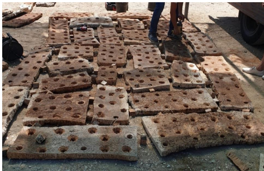
Figure 16. Laying out cork pieces on land during construction process (picture taken by author on 26.07.2022)
